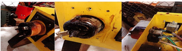
Example of fire hazard from plugging in heater
